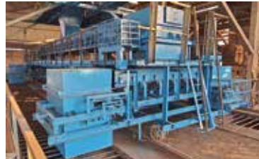
Shuttle Trolley with Conveyor
